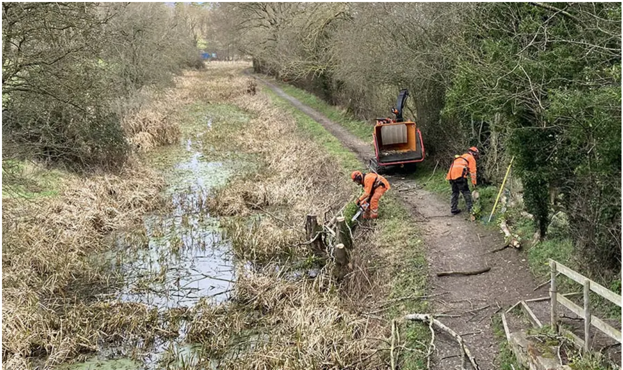
Workers cleaning overhanging tree branches on a section of the Montgomery canal. Photo: Canal & River Trust.
